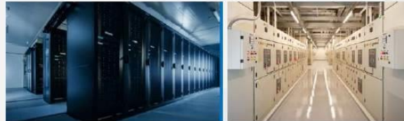
DATA CENTER DESIGN & INSTALLATION
